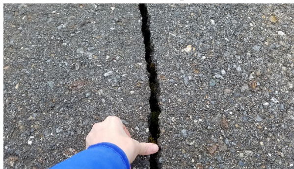
Exhibit 5-1: Asphalt cracks in known release area at north end of runway 02/20.
